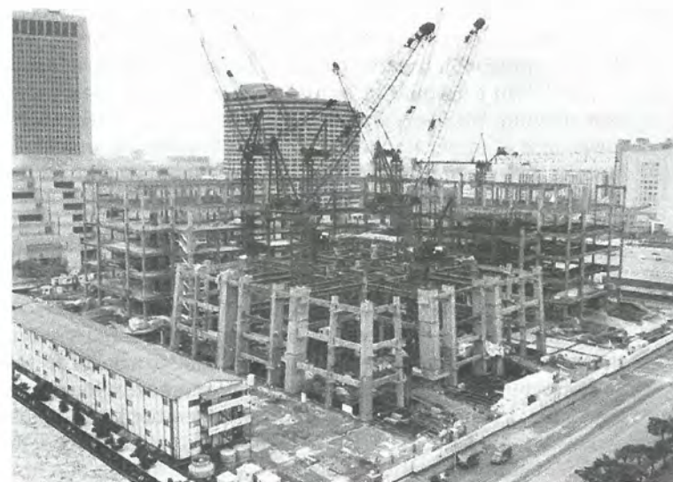
FIGURE 5.2 Construction photo during erection of the lower portion of the tower shows multiple cranes for tower and podium, two supercolumns on each face, and two supplementary supercolumns on each face.
